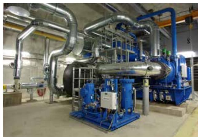
Helsinki’s Katri Vala heat pump captures heat from the city’s waste water.
