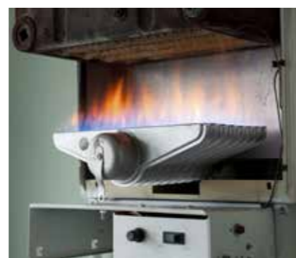
Individual air-conditioning units (top) and gas boilers (bottom) are just two of the technologies that district energy can replace.
