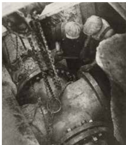
Installing a two-metre-diameter steam pipe for district heating in New York in the early 20th century (left).
