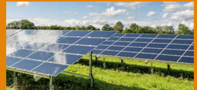
Solar photovoltaic panels in a field in Bavaria, Germany.
