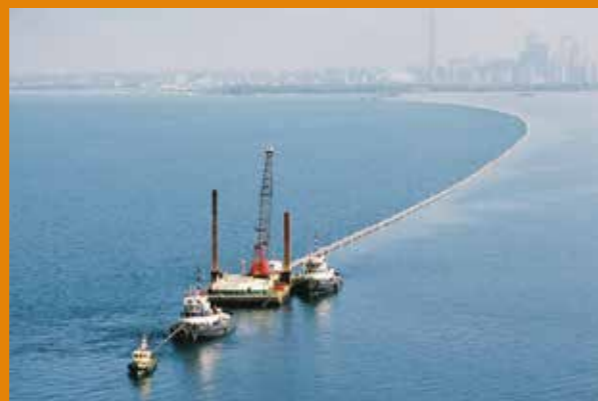
Toronto's deep-water cooling system captures cooling from Lake Ontario (see case study 3.5).
