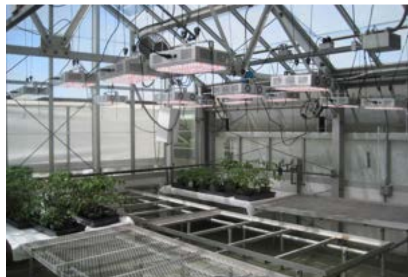
Photo: Department of Biology greenhouses were outfitted with efficient LED lighting under the ERP program, saving 248,000 kWh/year
