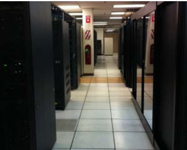
Photo: Data center end-aisle isolation
