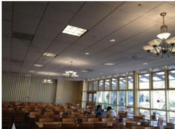
Chandeliers in Wilbur's main eating area have been retrofitted with LED lamps.
