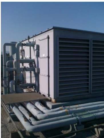
Before- Existing lab air handler
