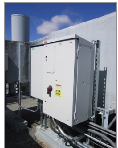
After- Existing lab air handler with VFD
