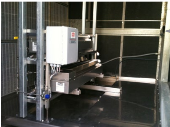
New electric ultrasonic humidifiers use less energy than steam units
